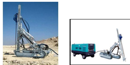
Gambar 3. Alat pemboran batukapur jenis Rock drill PCR300 & HCR1500 dan compressor airman PDS750S
