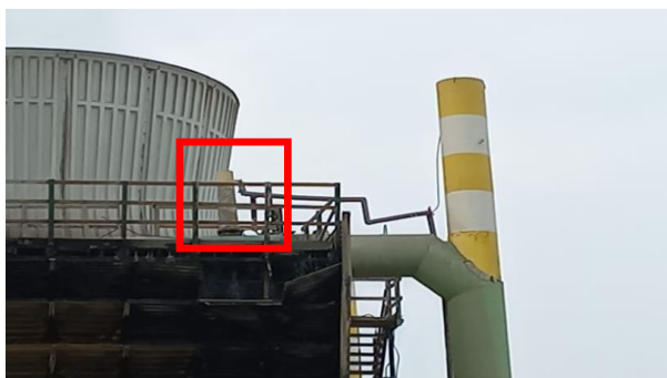
Gambar 4 Vent stack hot water return di unit Cooling Tower 4O-4204-U (area kotak merah).
